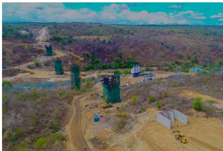
A view showing pillars whose construction has been completed at the New Wami Bridge in the Coast Region.
