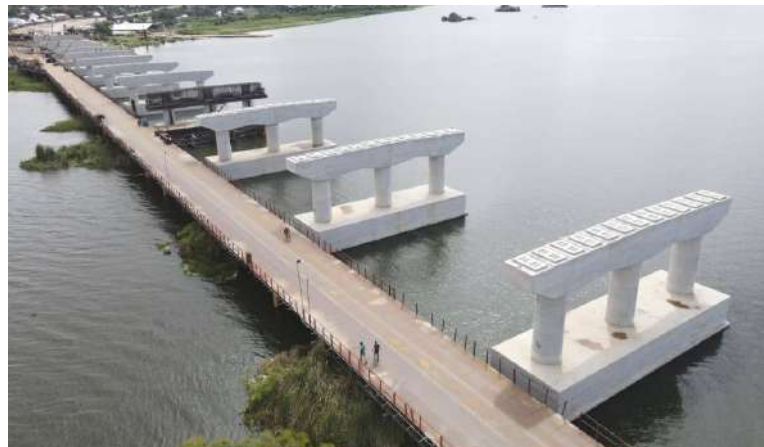
The construction of JP Magufuli Bridge (kigongo – Busisi), in Mwanza region now reaches 72 percent.
