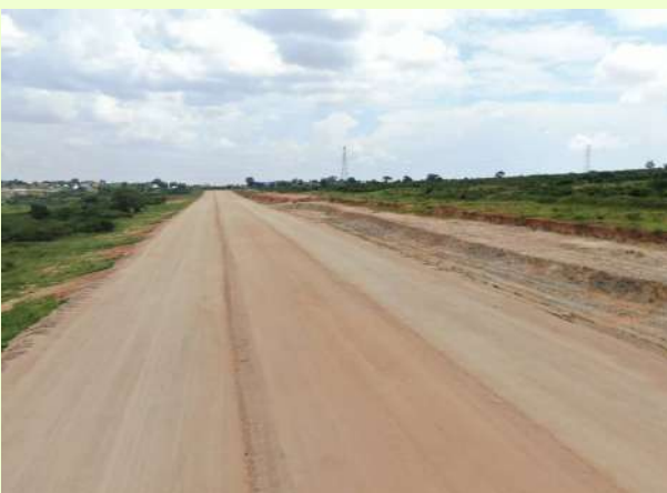
A section of the second phase of the Dodoma outer ring road under construction covering 60 km, and is expected for completion in March next year.
