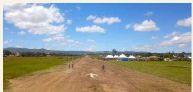
Part of the 1,750km 30metres wide Sumbawanga Airport runway in Rukwa Region undergoing expansion to tarmark level.
